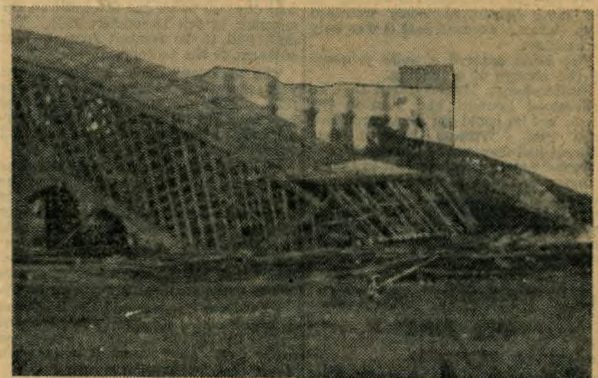
Collinstown Aerodrome, taken after its collapse recently.
