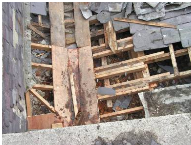
The new plywood gutter and valley boards. Note the reinforcement of existing timbers where they had rotted at the lower ends
