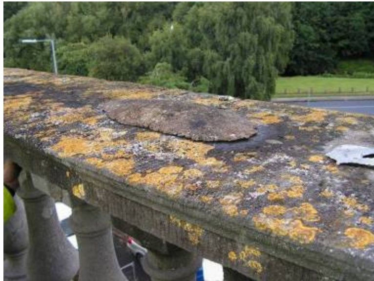
Some of the limestone cap stones on the north-east façade. Note the mortar covering or protection over the iron cramps which reinforced the most of the joints between the cap stones. Note also the tooled lines on the cap stones
