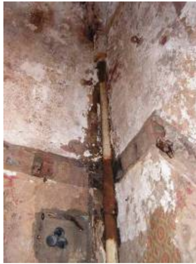
The corroded rainwater down-pipe in the southern lodge. Note the hole at the top of the pipe. Note also the joist holes in the brickwork which one supported the floor. Note the springing of the vault above.
