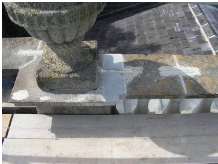
New limestone indented above the balustrade on the north-eastern façade. Note also the new stainless steel cramps
