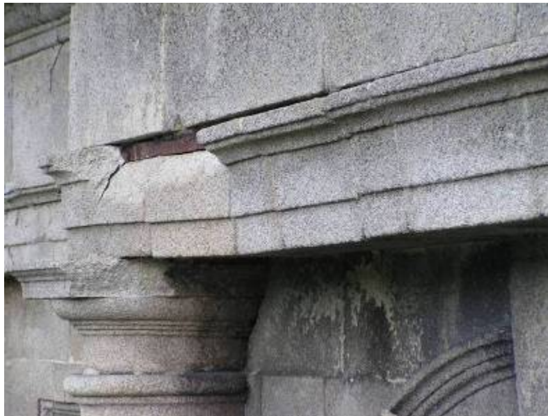
The same architrave of the north-eastern entablature viewed from the north-east. Note the exposed iron tie bar.
