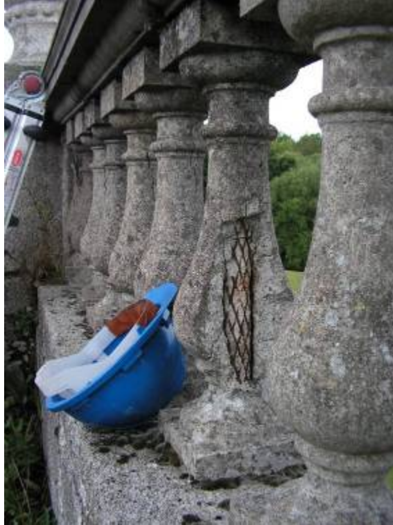
A baluster in the north-eastern façade, near the north-east corner. Note the corroded wire mesh reinforcement wrapped around a central iron or mild steel core and spalled, cast masonry.
