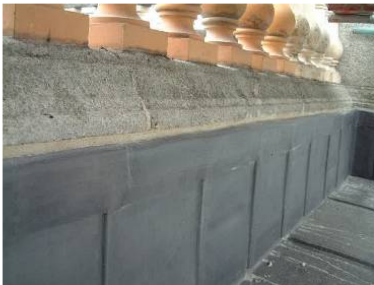
Pointing of cover flashings on the south-western blocking course with a lime mortar. Note the lead flashing built over the flaunching fillet and cornice as an additional protective measure.
