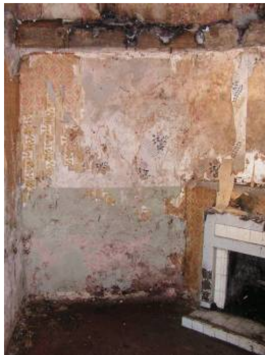
A view of the ground floor southern lodge. A small early 20 th century tiled fireplace is in the corner of each lodge; the flues ran up to the corner urns. Note the fragments of wallpaper on the walls; at least three separate papers were discernable, one has a decorative rose motif which probably dates from the early 20 th century. Note the fragments of the timber floor on the walls.
