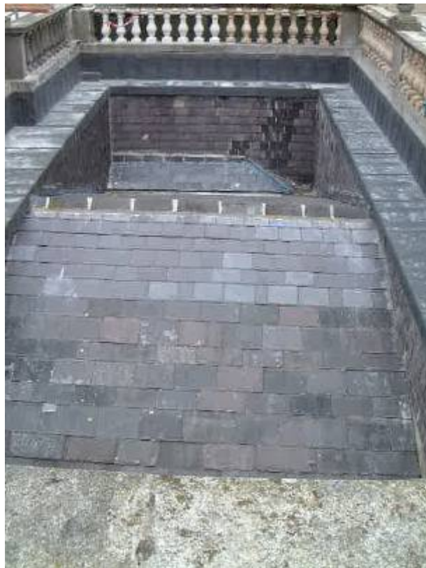
The repaired roof, viewed from the north-west. Note the darker, new vertical slate cladding. Note the lighter coloured slate on the 6 top courses of the roof slope and on the "small roofs" beside the valley.
