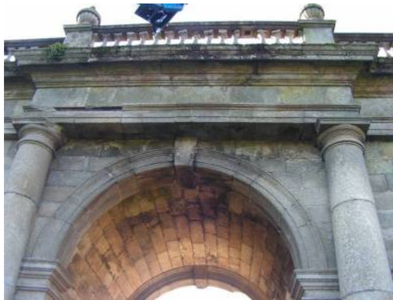
A closer view of the front of the central part of the north-eastern façade before works began. Note the missing piece of stone and the damaged and missing balusters (photographed January 2009)
