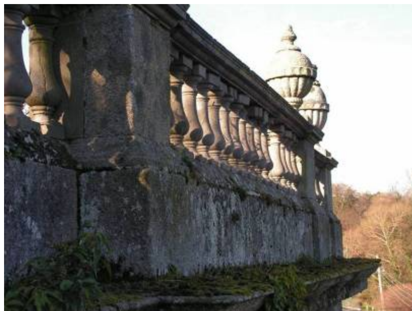
The upper surface of the cornice above the north-eastern façade. Note the extensive growth of mosses and weeds on the flat surface. (photographed January 2009)
