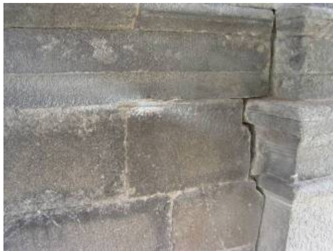
The south-eastern façade: the repaired stone and re-pointed mortar joint after the steel plate had been drilled out.
