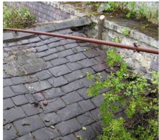
The hole in the roof and shrubs growing from it
