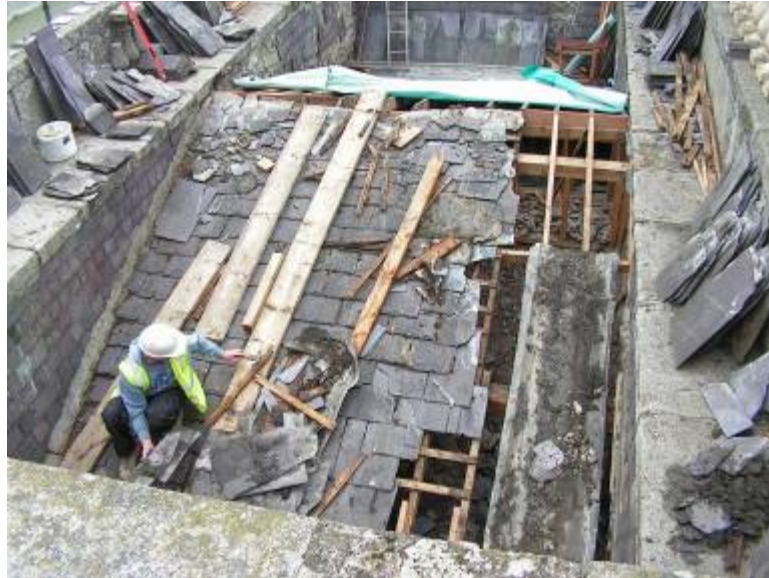
The roof repairs underway, viewed from the north-west. Note the balustrade on the north-eastern façade had been mostly taken down
