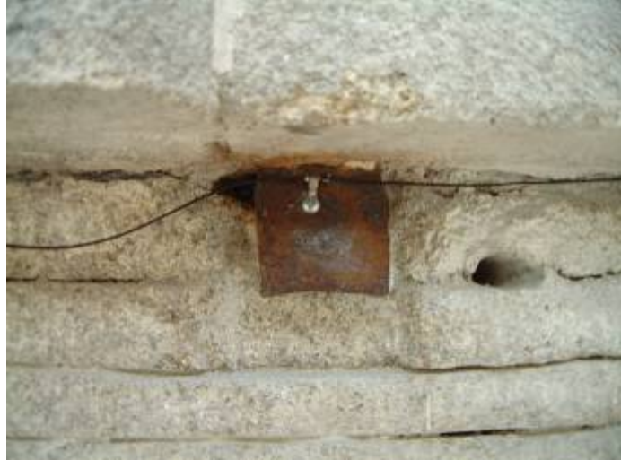
The lower frieze of the south-western façade: the end of an iron cramp to which a cable has been connected. Note also the chipping of the stone and dowel hole which will act as a key for the mortar behind a new stone indent in this area.
