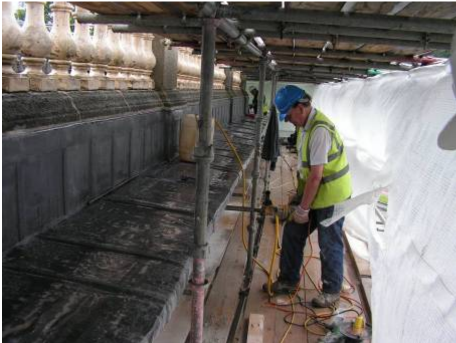
Drilling the cores at each joint in the corona course of the south-western cornice to each cramp behind to allow the cables to be attached to each cramp.
