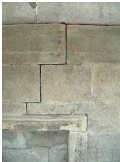
The north-western façade: chase cut into the mortar joints to accommodate the cable, part of which is visible.
