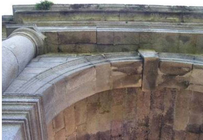
The damaged projecting entablature on the north-eastern façade viewed from below. Note the crack on the underside of the architrave of the entablature, the damaged capital & plant growth on the cornice on the left in the image. Note also the green lichens and black stains left by water run-off and residual dirt and salt staining.
