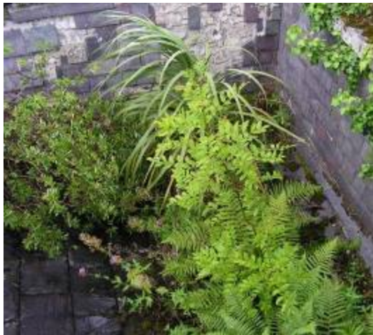
Biological colonisation of the northern gutter
