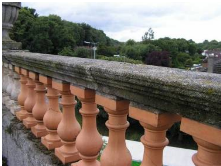
Some of the granite cap stones on the north-western façade. 3 of the 4 facades had granite capstones. Unusually this balustrade had only 2 iron cramps (visible at the far end) and the sectional profile was slightly thicker than elsewhere
