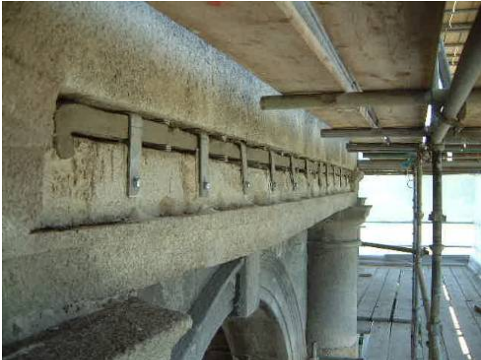
The north-eastern entablature: the exposed iron beam with the stainless steel L-sections bolted to the stone blocks below and hooked over the iron bar above. Note also the stainless steel shims or packers above and below the iron bar.
