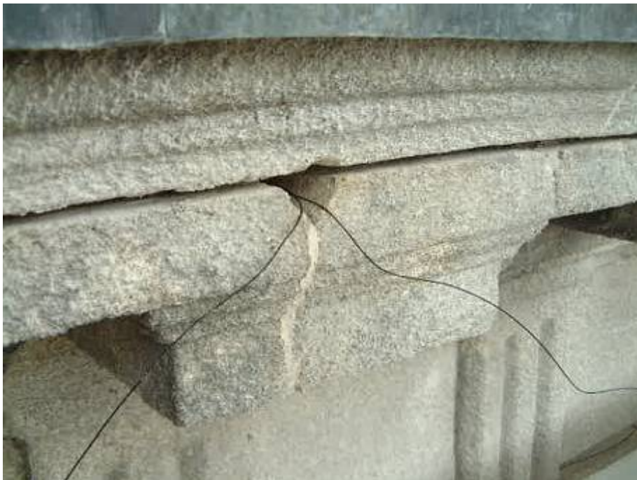
The south-western cornice: core hole drilled into the joint between the corona and mutele courses
