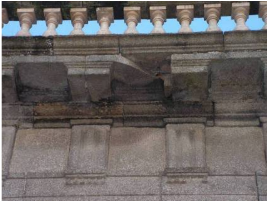
A closer view of one part of the damaged dentil course of the south-western façade. Note the small piece of cramp visible
