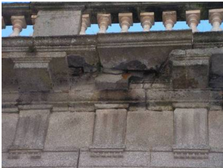
Another part of the damaged dentil course of the south-western façade. Note the slightly jacked stone at the top of the cornice and the edge of an iron cramp at the back underneath. Half of another cramp is visible on the left. Note the iron oxide stains.
