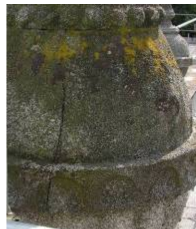
Crack in the large flue-urn at the north-eastern corner
