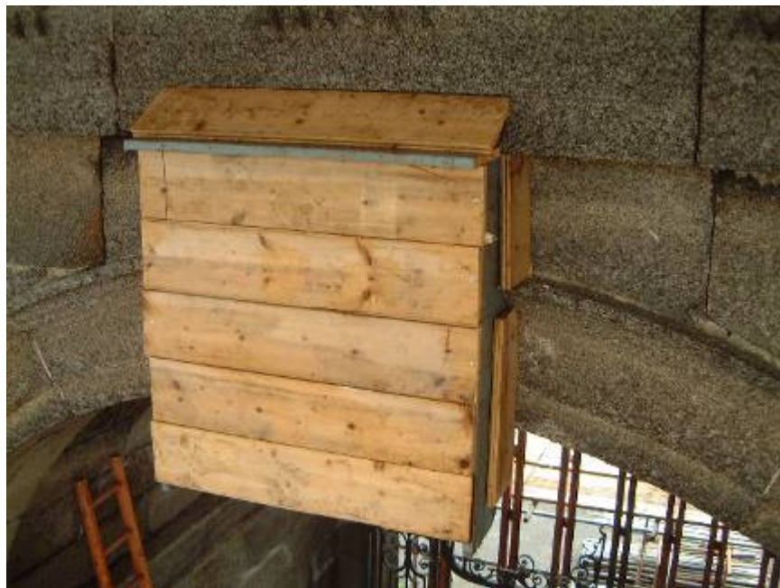
Protection of the Coade stone mask from damage during the works. A silicone cast was also taken of the mask to help reconstruct it should it be damaged during the course of the works
