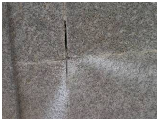
The north-eastern façade: a close up view of the left-side, square recessed panel where a pin, approximately 200mm long, was drilled out of the stone. Note where the stone had been drilled out around the pin. The resultant cavity was filled with a mixture of granite dust and resin, into which a chase was made while still fresh aligning with the mortar joints. The resin-dust repair was then tooled to match the appearance of the surrounding stone during dry weather conditions.
