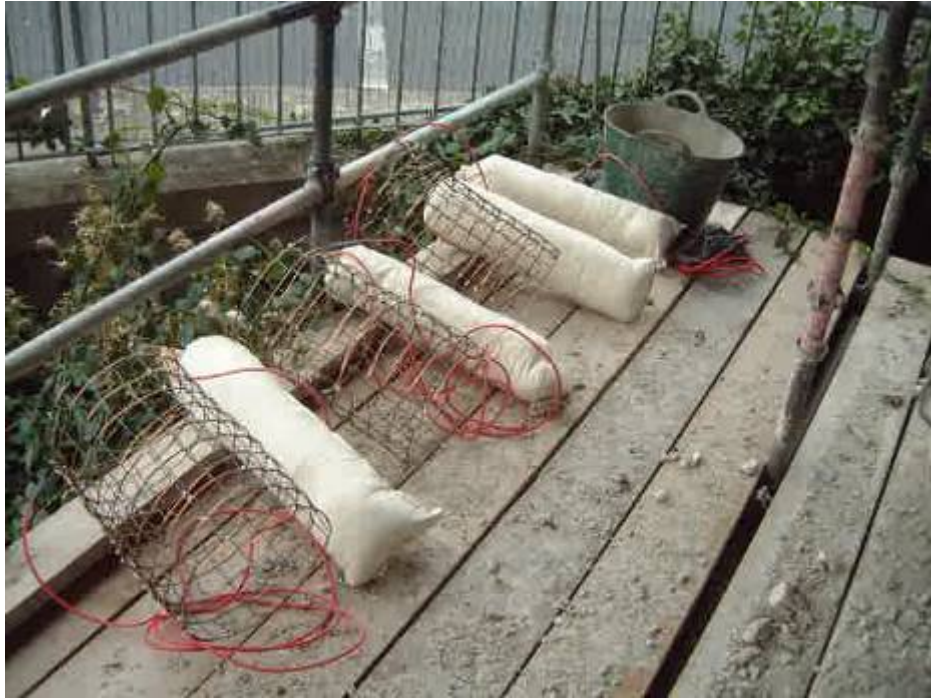
The 4 magnesium anodes, approx. 700mm long before they were placed in the 4 holes behind the northern flanking wing wall
