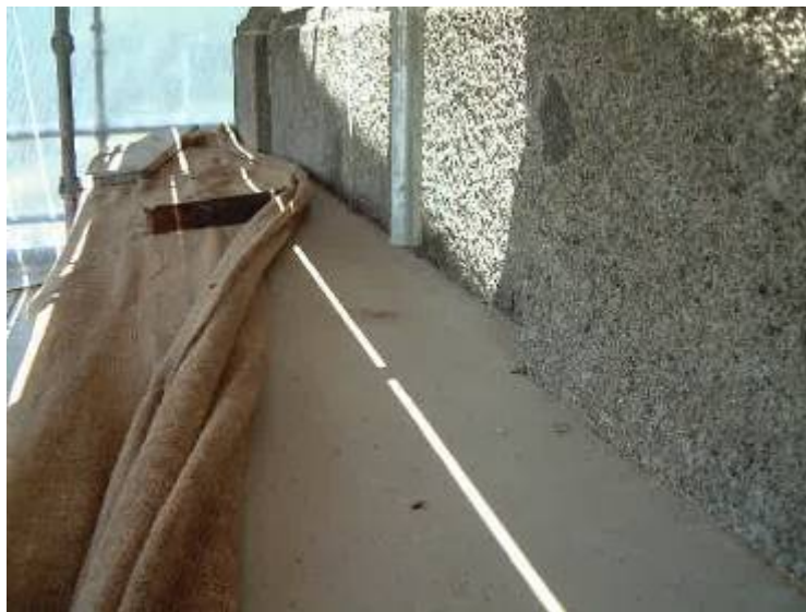
The lime mortar flaunching fillet on the cornice, protected with dampened hessian after its application.
