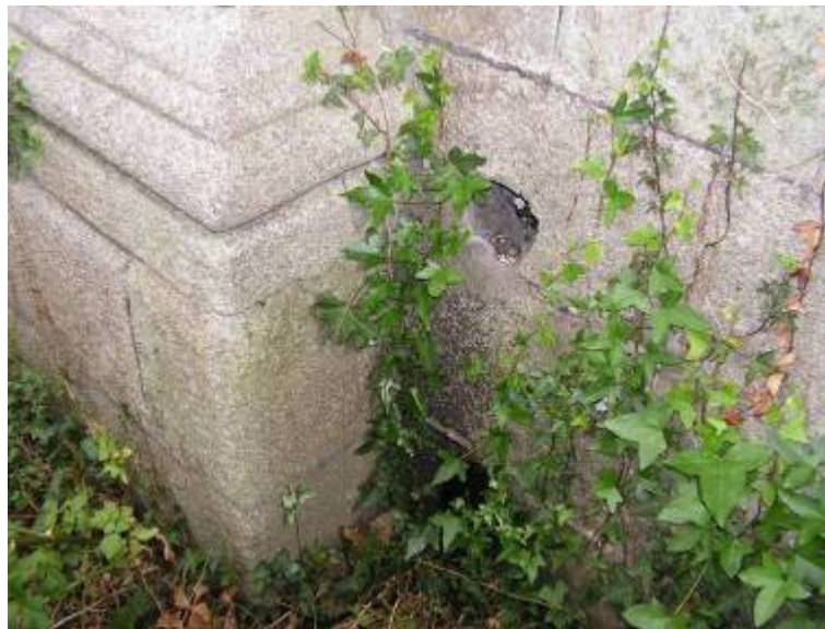
The rain-water outlet from the southern lodge, at the base of the south-eastern facade. Both outlet pipes had badly corroded within the stone opening causing localised damage in the area.
