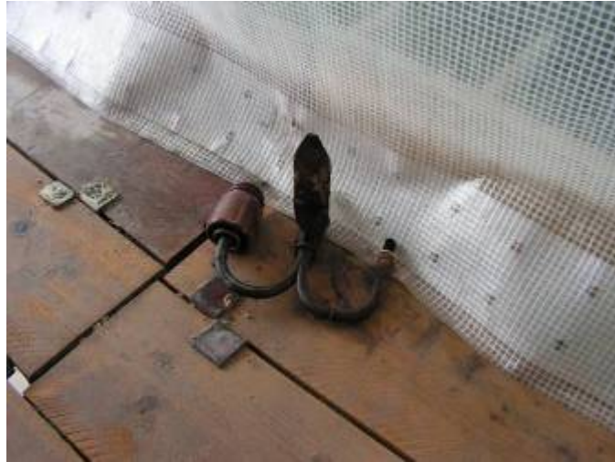
An old electrical supply point which was partly built into a mortar joint in the south-eastern façade.
