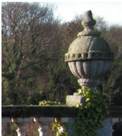
Crack in the southernmost smaller urn on the south-western façade
